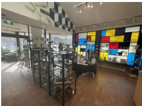
Out with the old...a final picture of the Gift Shop before demolition began on April 25th.
